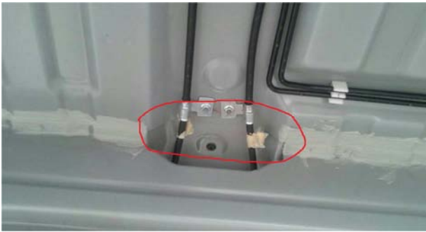
Figure 10. Leaking glue under the floor.
