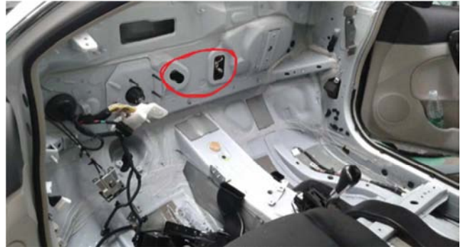
Figure 8. Water inlet at the through-hole position of air conditioning pipe.
