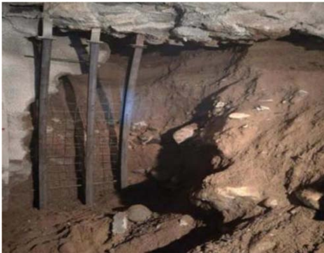
Figure 2. Steps collapse in tunnel excavation.
