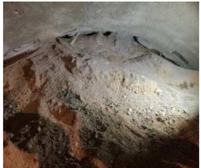
(a). Arch collapsed.
