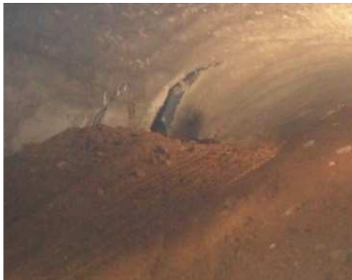
(d). The initial supporting cracking.
