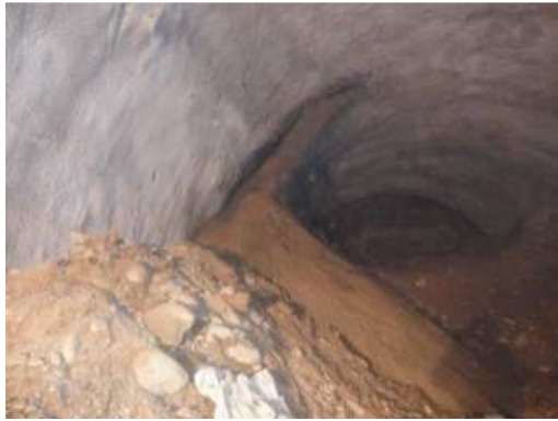
(c). Hance collapsed.
