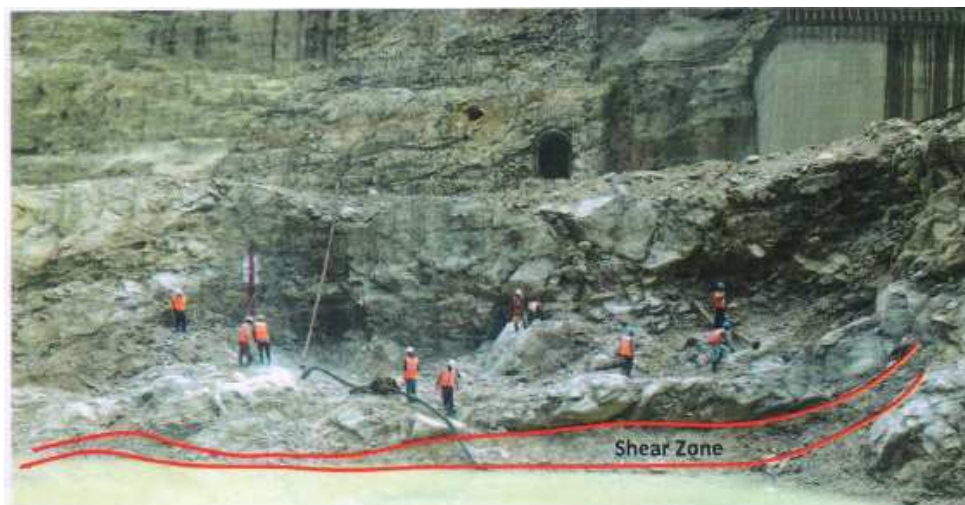
Figure 3. Shear Zone Right Side of Excavated Trench.
