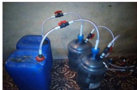
Figure 3. Biogas Digestion plant.
