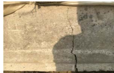
Figure 12. RC plate mid-span crack.
