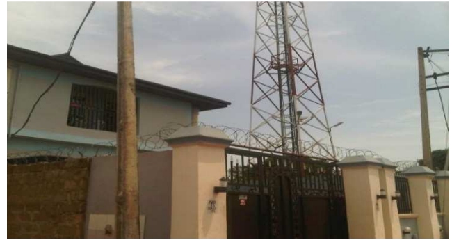
Figure 1. b. A snap shot of assessed base station site at 1 st Ughor.
