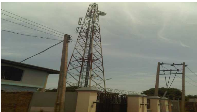
Figure 1. a. A Snap Shot of Assessed base station site at Alyanyo street.
