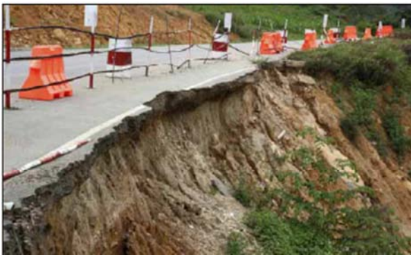
Figure 12. Geological hazard safety monitoring.
