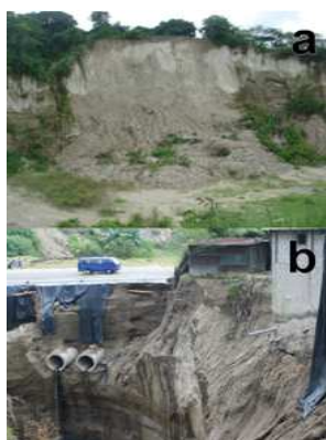
Figure 1. Mass wasting problems in Tierra Blanca Joven (TBJ). a) corresponds to las Cañas River where mass movements, erosion and collapse occur all the year. b) Is a 2005 photo of a stream in Ilopango, the landfill and pipelines of the road failed during heavy rains of hurricane Stan.
