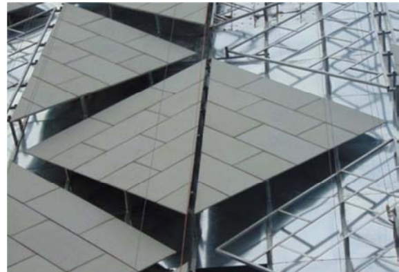
Figure 8. Picture of installing process of composite stone simply supported on four sides.
