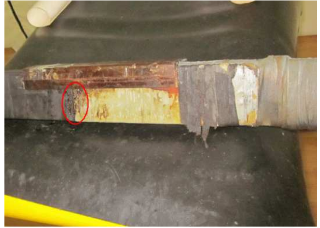
Figure 2. Stator winding insulation failure.
