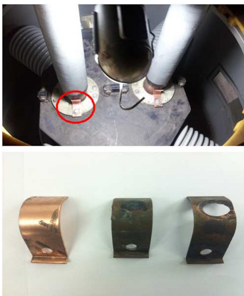
Figure 10. Gap discharge location.
