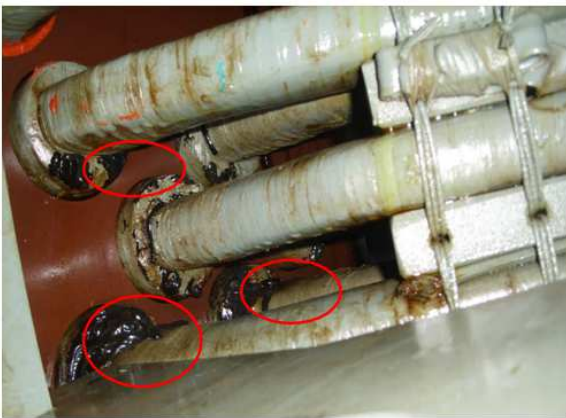
Figure 1. Compound melting due to overheating.
