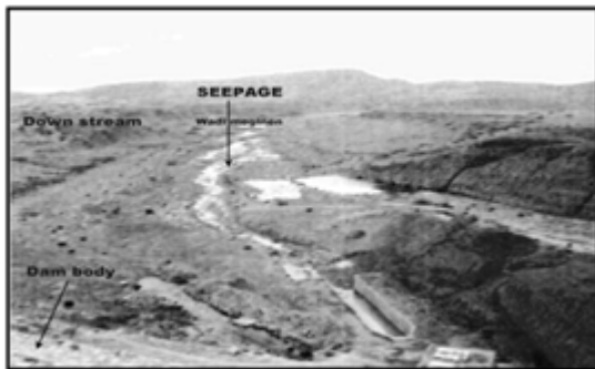
Figure (4): seepage phenomenon downstream of the dam
