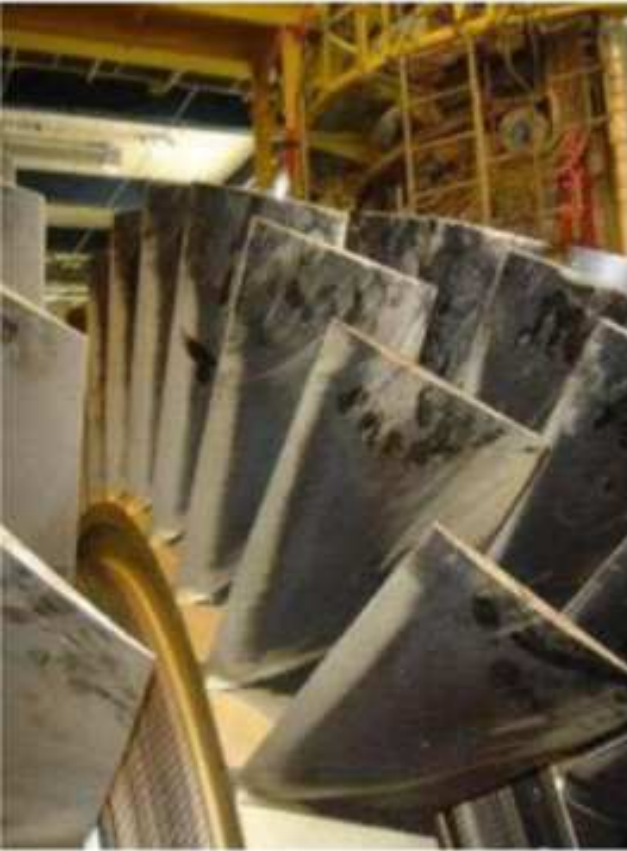
Figure 1. Example of fouling particles that attached on the airfoil of compressor blade [21].
