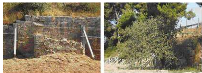
Figure 4. A anti-aesthetic retaining stabilization system with metallic pillars at the existing part of the ancient wall of Olympia.
