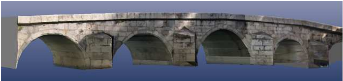
Figure 3. Wireframe 3D model created with photogrammetric process. a) Upstream side, b) downstream side.
