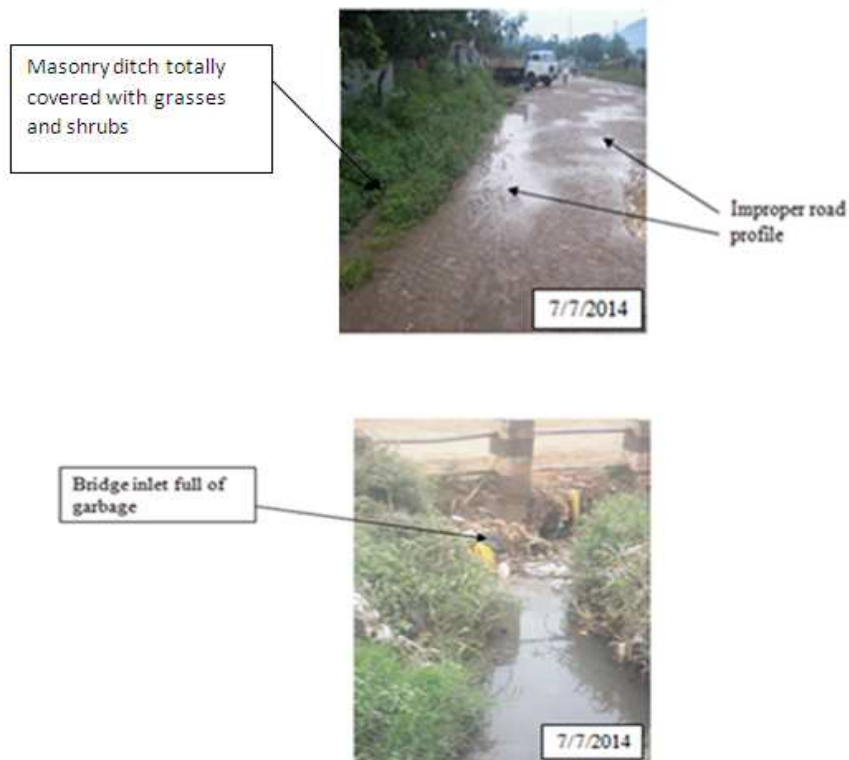
Figure 9. Poor maintenance of drainage ditch, bridge and road surface.
