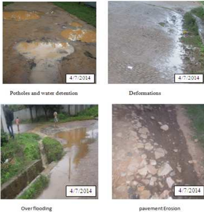
Figure 7. Photo showing Road damages of the study area.
