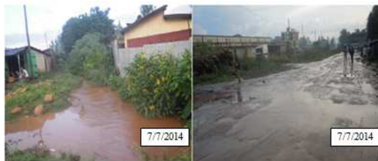
Figure 10. Over flooding of road due to bridge and pipe culvert blockage by debris.
