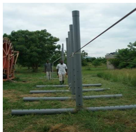
Figure 1. Perforated uPVC pipes.
