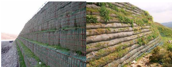
Figure 7. Examples of using soft views. (Right) step (from: www.retainingsolutions.com.au ) (Left) vertical (from: www.akturkinsaat.com.tr )
