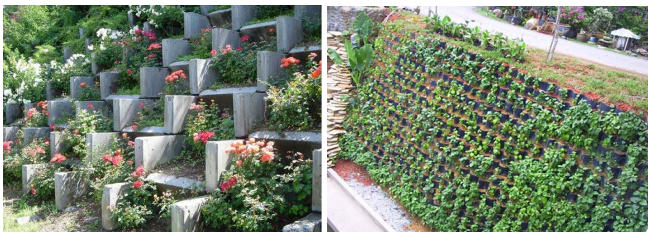
Figure 8. Examples of compound views (Right) the use of concrete blocks (from: khakemosalah.ir ), (Left) the use of plastic baskets (from: www.miracell-ccs.com )
