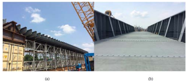
Figure 15. (a) Floor beams before receiving second girder, and (b) view of span 2 with all knee braces installed.
