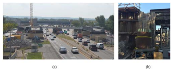
Figure 17. (a) Situation prior to super weekend and (b) Wire sawing of south abutment.
