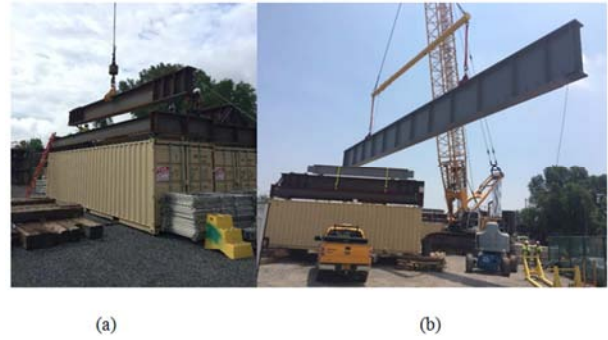
Figure 14. (a) Grillage steel positioning on connex box, and (b) setting of the first girder for span 2.
