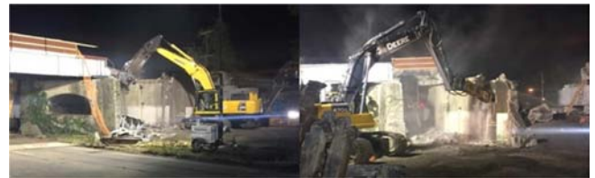
Figure 19. Demolition process: Shearing down the existing TSR Bridge deck (left) and Hammering out the existing abutments (right).
