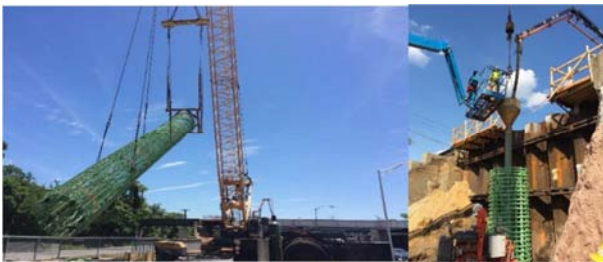
Figure 5. Transportation of the rebar cage with picking ring (left) and placing tremie with pump truck (right).
