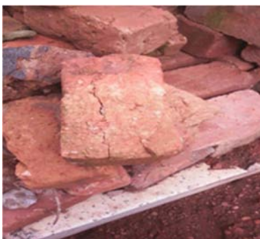
Figure 2. Cracks and breakage.
