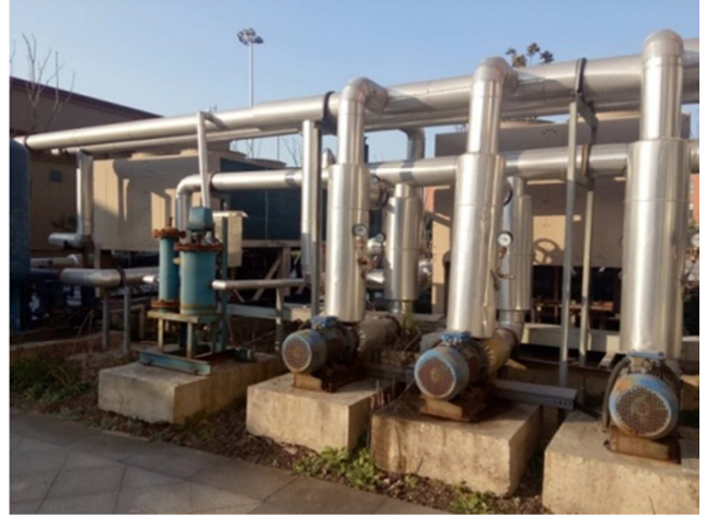
Figure 1. Central air conditioning environment.
