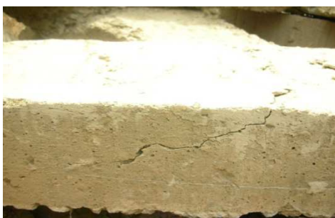
Figure 7. Crack Failure of Beam
