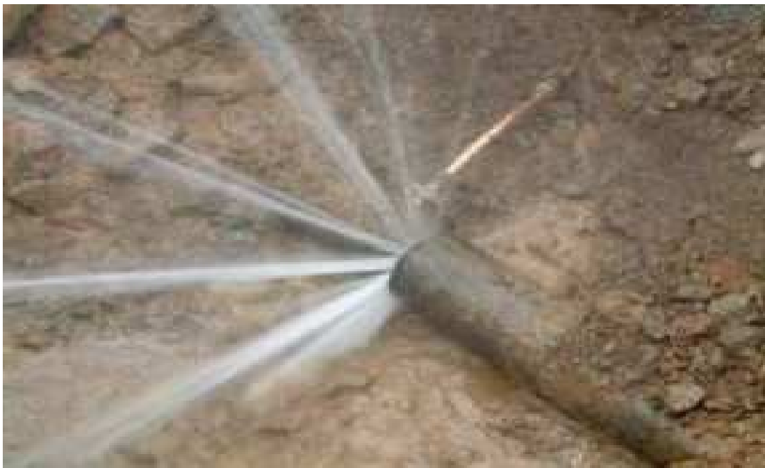
Figure 3. Pipe Bust Due to High Pressure in the Water System.
