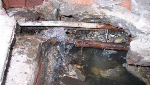
Figure 4. Aged Water Pipe Broken.
