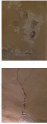
Figure 4. In these pictures, it is possible to recognize the detachments and the lesion visible in the internal part of the church, corresponding to the area in which the GPR survey is acquired.
