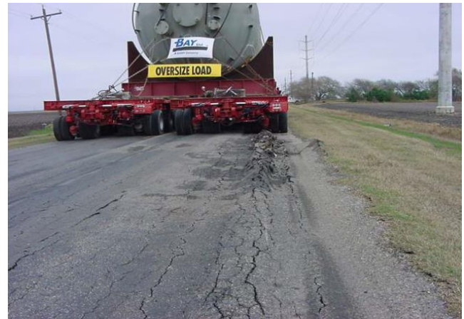
Figure 1. Severe pavement damage on pavements by SHL movement [6].
