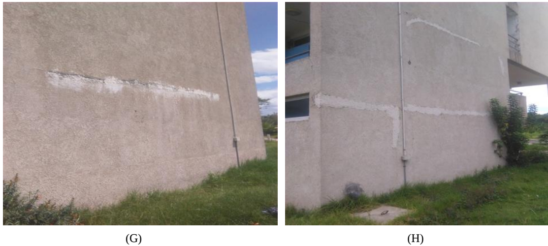
Figure 3. Ad hoc crack repair using cement paste, without prior crack-type diagnosis (G–H).
