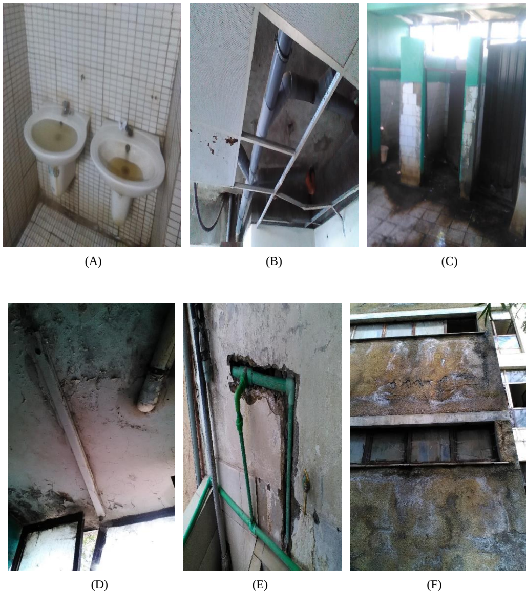
Figure 2. Sanitary and building-fabric deterioration in male dormitory blocks (A–F).
