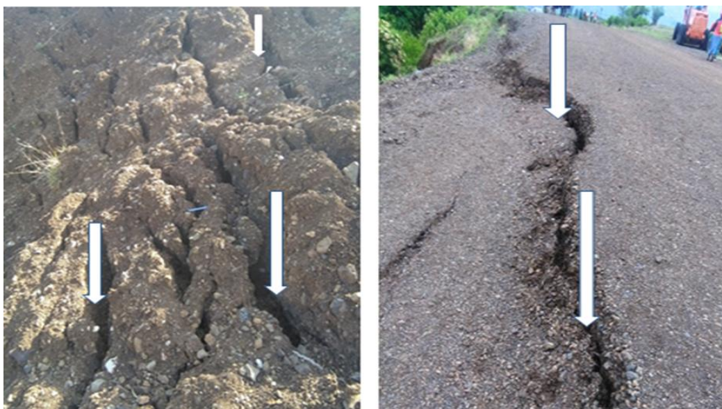
Figure 6. photo shows tension crack along road Gidole – Wozeka.
