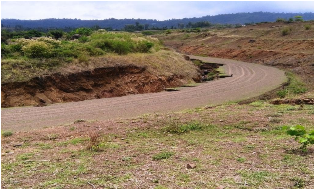
Figure 11. Damaged roads by landslide.
