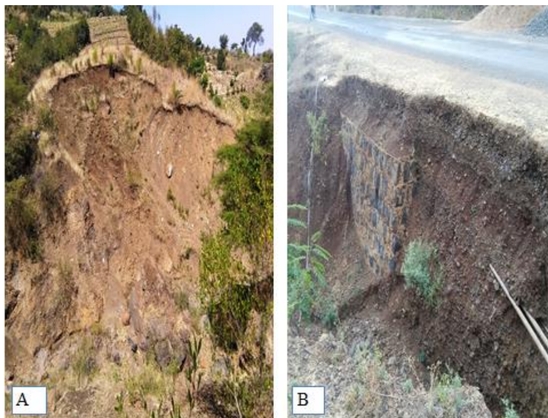
Figure 13. A Damaging farmland. B, Damaging of pipe line, retain wall and road under risk.
