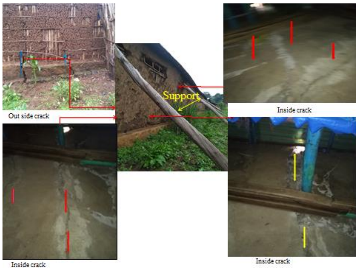
Figure 12. Police station that under risk and different cracking inside and outside of house.
