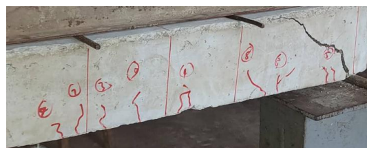
Figure 9. Visible Cracks on Concrete Beam During Flexural Strength Testing.
