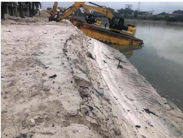
Figure 4. Slip failures in formed sand slope.
