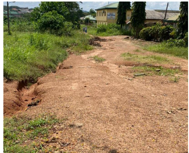
Figure 7. Condition of Road at Middle Belt of the Campus.
