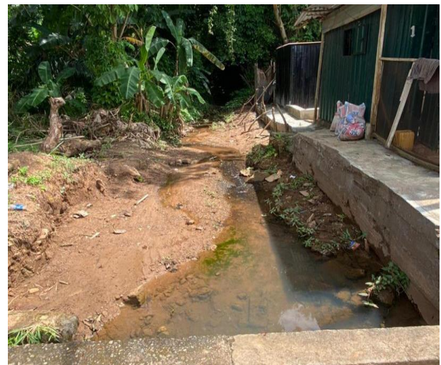
Figure 6. Drainage Condition at Maintenance Are.
